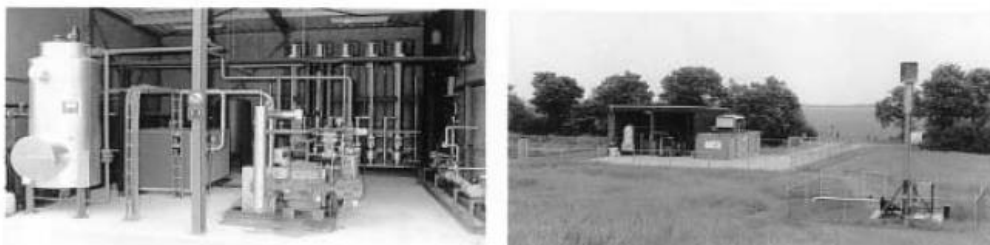
The Example of the Separating Carbon Dioxide Membrane System placed in the Garbage Reclaimed Land
