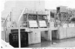
제강설비 Screening equipment (Trash take)
