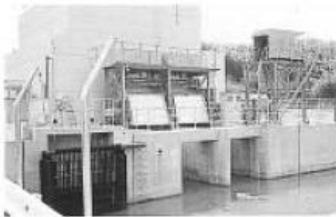
Screening equipment(Trash rake)
