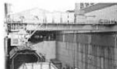
Overhead travelling crane
